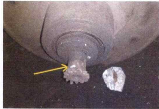
Figure 5: Worn-out Pinion of driving motor
